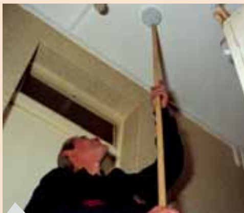
Photo: London Fire Brigade Aiming high: Community Fire Safety work is paying dividends in London.
